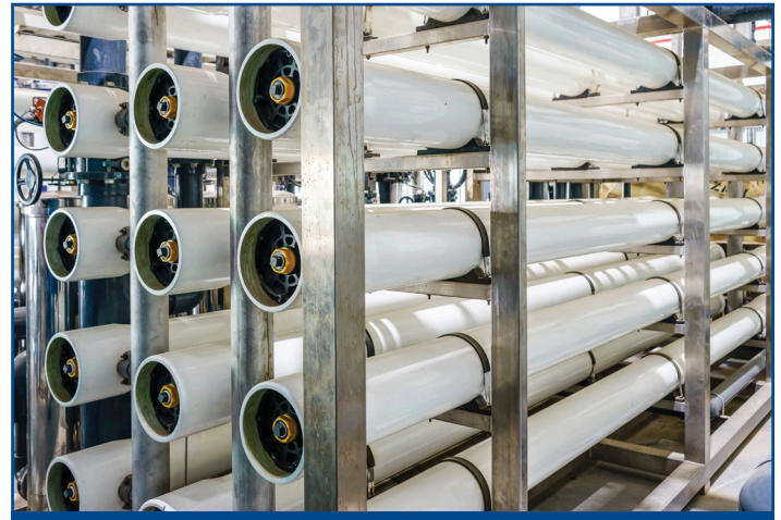
Figure 2 RO Membrane System in Utilities Water Production
