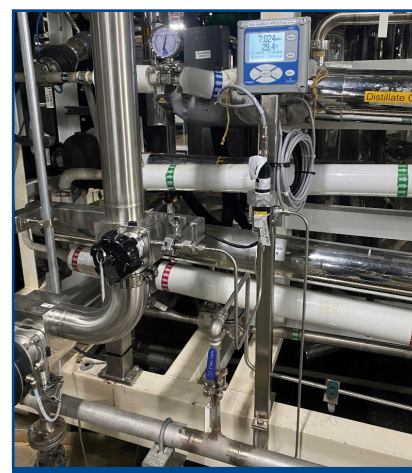
Figure 3 WFI Generators at Novartis in Singapore. Permission granted for use by customer.
