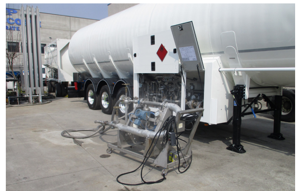
Technoimpianti calibration bench, used to test flowmeters installed onboard of trucks
