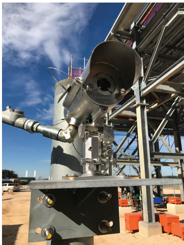
Figure 3. An open path combustible gas detector can detect a cloud of gas moving through its beam, even if it has diffused to a relatively low concentration.
