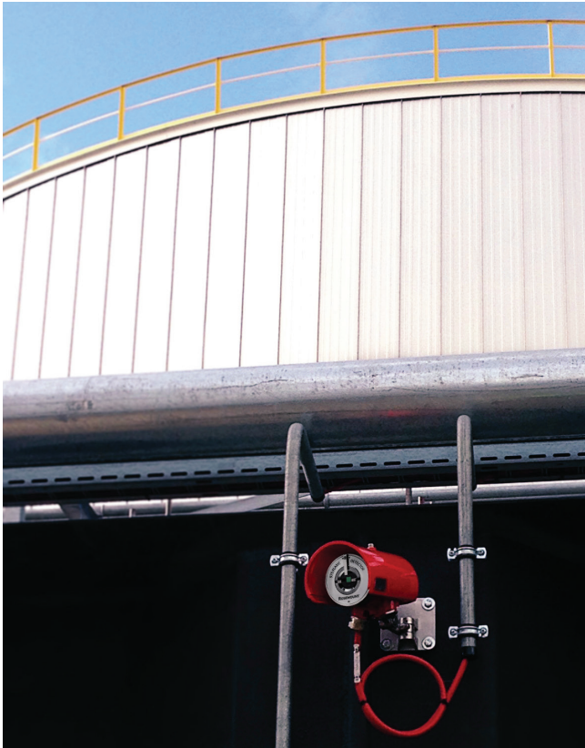
Figure 4. Flame detectors look for radiation in specific wavelengths emitted by hydrogen- and carbon-based combustion.
