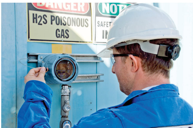
Figure 2. This type of fixed-point combustible gas detector can detect a wide variety of flammable gas types with percentage of lowest explosive level measurement.
