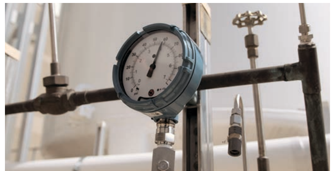
FIG. 1. A proprietary wireless pressure gauge ® does the same job as the mechanical version but with multiple advantages.
