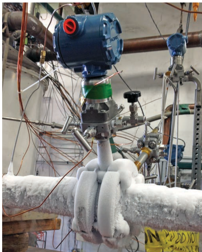
FIG. 7. DP flowmeters can be used with LNG and other cryogenic liquids, but the transmitter should be placed above the pipe.
