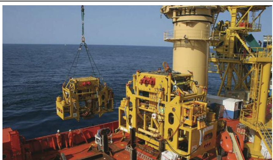
Three subsea multiphase pumps installed in almost 5,600 feet of water at BP’s King Field have a tieback distance of 20 miles and total capacity of nearly 75,000 barrels a day at a gas volume fraction of 98 percent.
