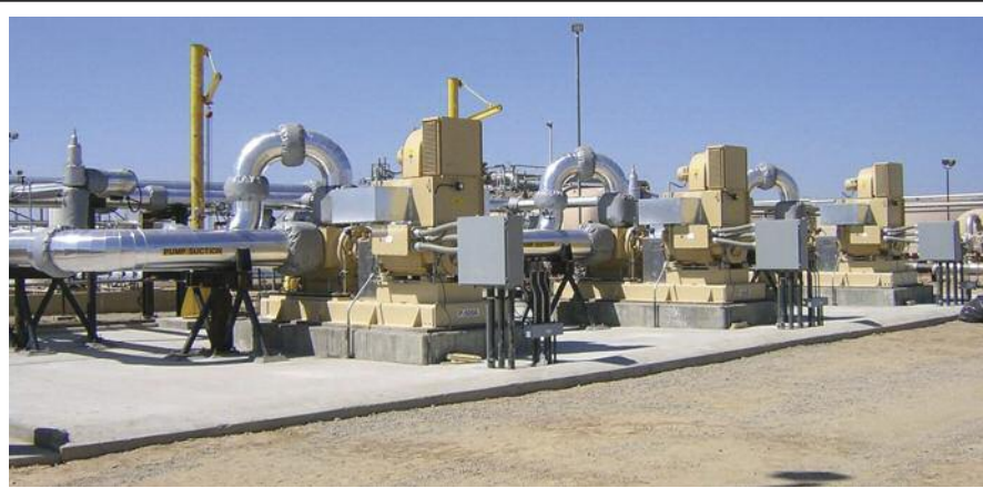
Aera Energy has three multiphase pumps handling 1,000 wells producing heavy oil using a combination of steam flooding and multiphase pumping at its Belridge Producing Complex in California.
