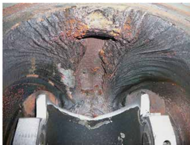
▲ Figure 2. Valves can fail where erosive or corrosive fluids are present. In this example, erosion damage occurred on the outlet of a separator inlet control valve in a coal seam gas application. Erosion was caused by the valve being oversized and operated barely open, coupled with poor material selection unable to withstand erosion from entrained particles.
