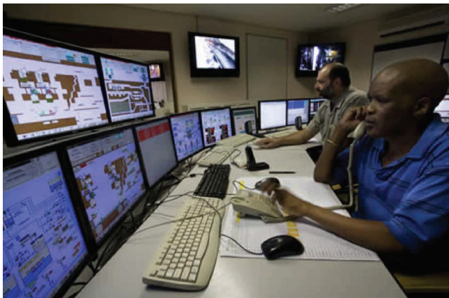
Figure 1. A centralised pipeline monitoring system relies on data that sometimes is sent from thousands of miles away.
