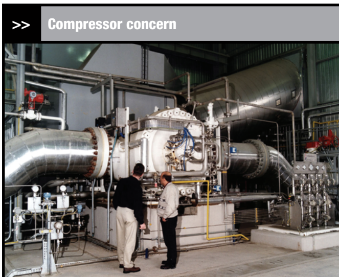
Figure 1. Fouling due to the rapid build up of deposits causes compressor performance to suffer.
