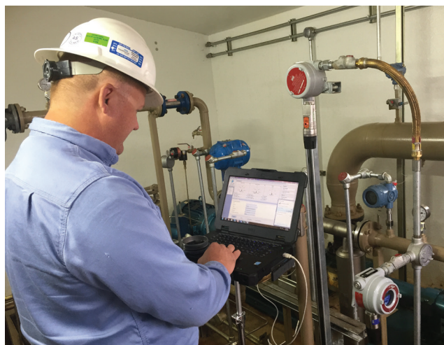
A service technician performs meter verification.
