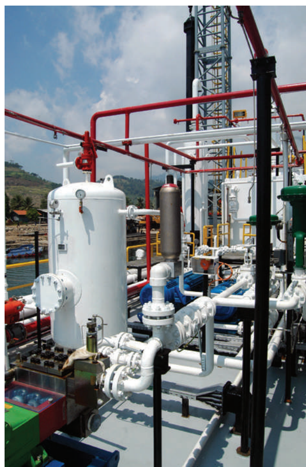
Fisher control valves shown in an offshore environment.
