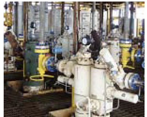
Temperature monitoring for 16 wellheads is done with nonintrusive, flexible pipe clamp sensors.
