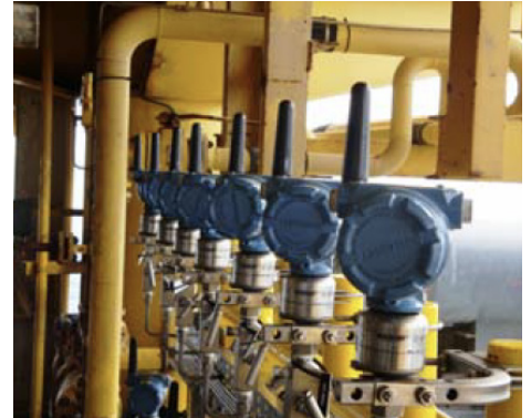
Casing pressure monitoring on 16 wellheads
