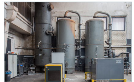
Compressors and compressed air storage in the compressed air centre
