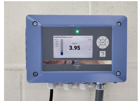
Image #2 The Rosemount 3490 Controller is installed indoors, and shows the wet well status in real time
