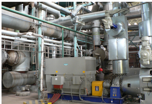
One of the installed new pumps with variable frequency drive.
