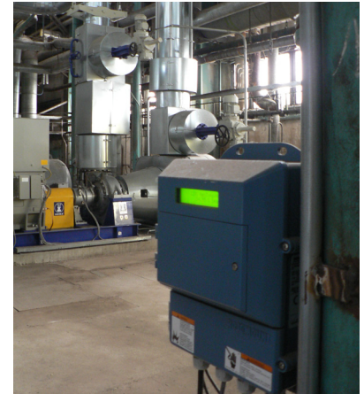
An installed Rosemount DN300/12-in. Magnetic Flowmeter to monitor the water flow and pump performance.
