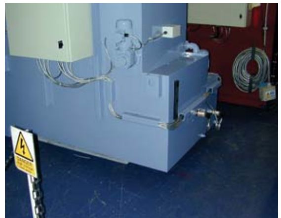
Two 2110 compact switches installed in a large filtration unit.
