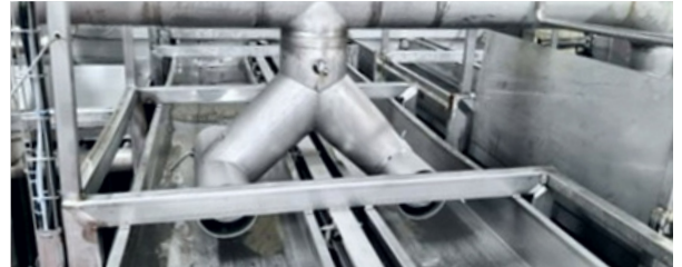
Brine sprinkler used on the tanks.
