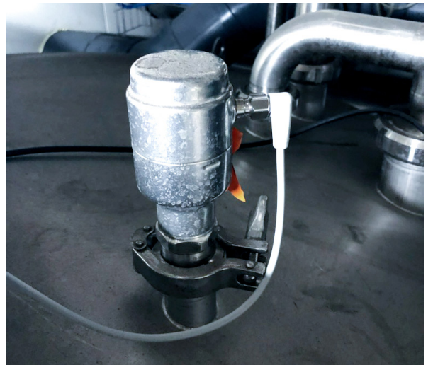
The Rosemount 1408H is installed on the brine tank.
