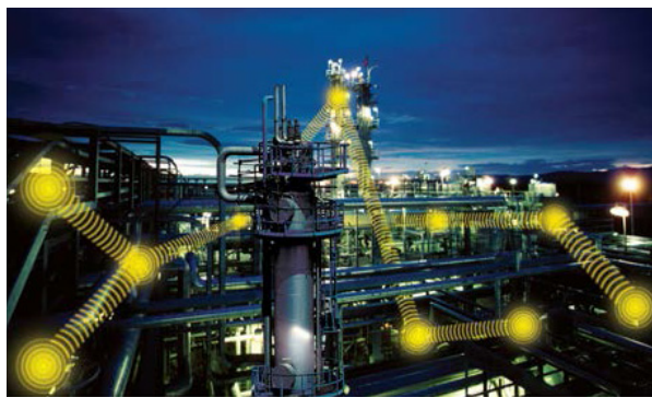
Emerson Smart Wireless Temperature Transmitters form a self-organizing wireless network across the Jubail plant.
