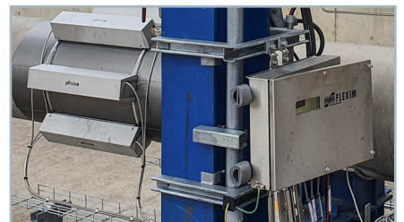
Measuring point with the stationary four channel FLUXUS® G706 ultrasonic flowmeter
