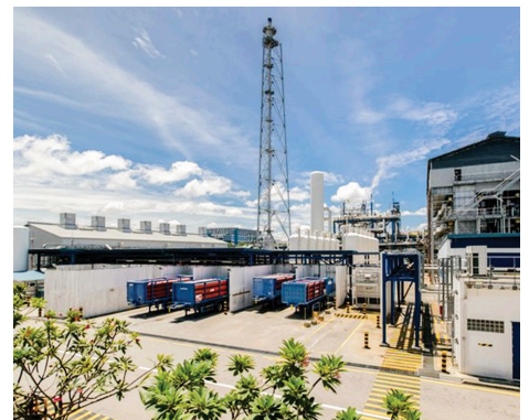
Image 1. An exterior view of a gas plant like the customer's site that would supply gases to the main plant from the utilities wing of the plant.
