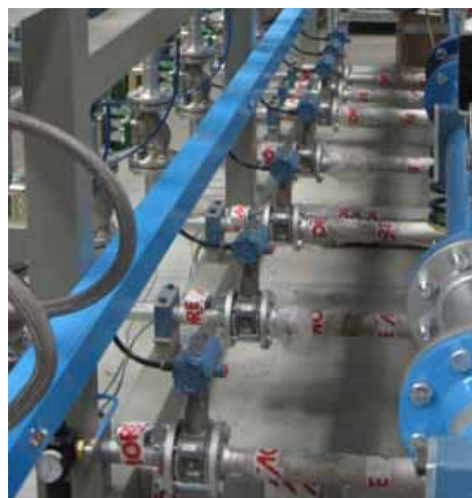
Installed Rosemount 8800 Vortex Flowmeters to control the injector feed of oxygen supply for a more accurate oxygen-fuel ratio.
