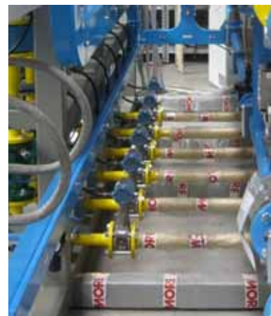
Rosemount 8800 Vortex Flowmeters installed to monitor natural gas flow.
