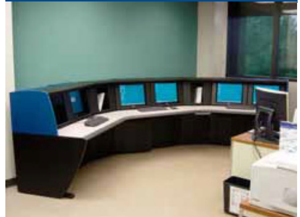
Dairyland's J.P. Madgett Ovation simulator mimics the control room layout to provide realistic training conditions for the plant operators.
