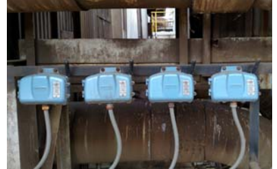
These transmitters were installed as a replacement for the 1000-Ft. 20 pair thermocouple cable that failed. Having the wireless system in place allowed for a rapid return to service without immediately replacing the cable.
