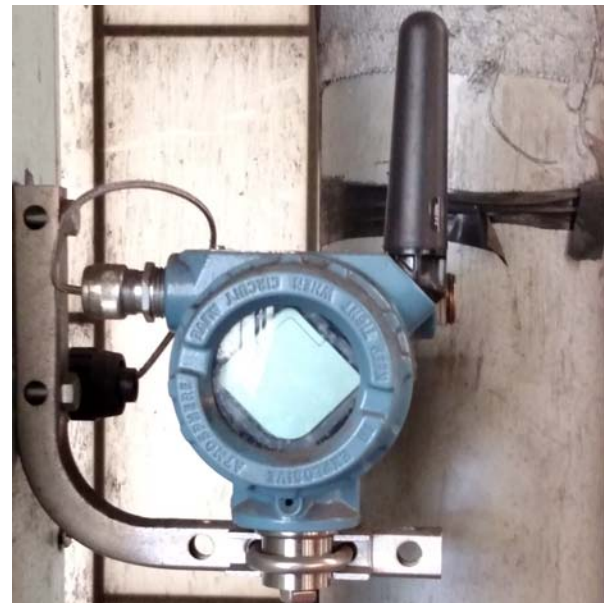
Rosemount 648 Wireless Temperature Transmitter measuring room temperature in the turbine house for freeze protection
