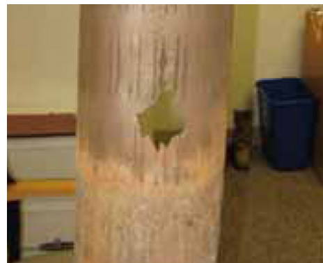
Cut liners from over-injection of steam is one of the hazards of poor steam injection control
