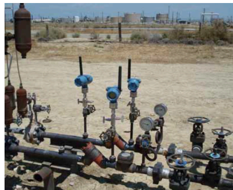
3051S WirelessHART™ pressure transmitters on a dual injection steam well.
