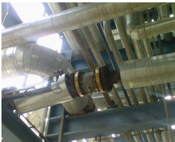
A Rosemount 8800 CriticalProcess™ Vortex flowmeters with the Severe Service Sensor for tough yet critical flow applications installed at the feedline.
