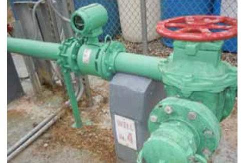
A Rosemount 8750W Magmeter installed in one of the water wells.
