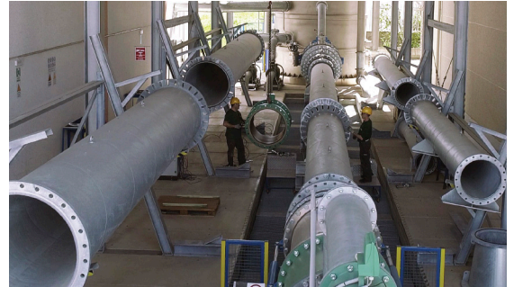
Extended line size Magnetic Flow Meter sensor installation.
