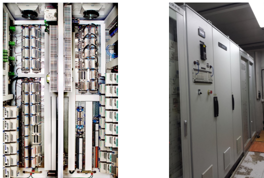
Ovation GE turbine control packaged retrofit of a Mark V system
