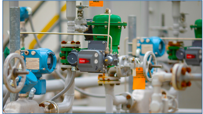
AMS Device Manager Data Server offers a solution to aggregate disparate and underutilized data from smart devices like control valves and measurement instrumentation, and further exploit it for positive impact elsewhere in the organization or technology stack.
